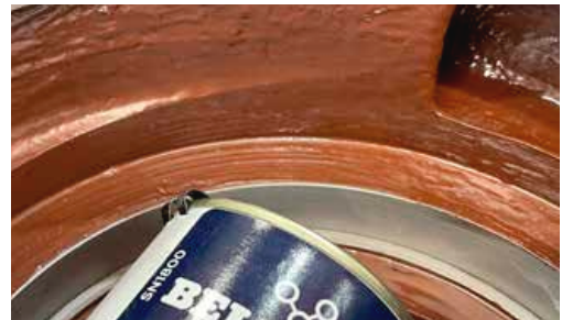
Disappointing repair reality – brushed-on epoxy ceramic. No engineer wants to see such turbulence-generating results anymore. Today, “good” looks fully different ...
